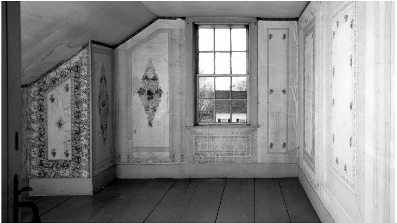
An attic room in the Field-Hodges House, November 1998. Panels and fragments of rare nineteenth-century wallpaper were intact throughout the room. Photograph by David Bohl. Courtesy of Historic New England.
