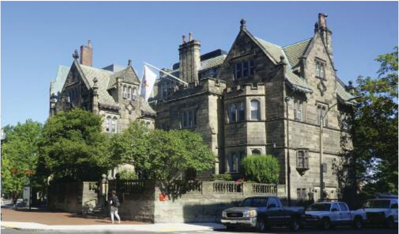
Exterior of “The Castle” before restoration, 2015. Damage to the exterior masonry from erosion and urban pollution required a comprehensive assessment.
